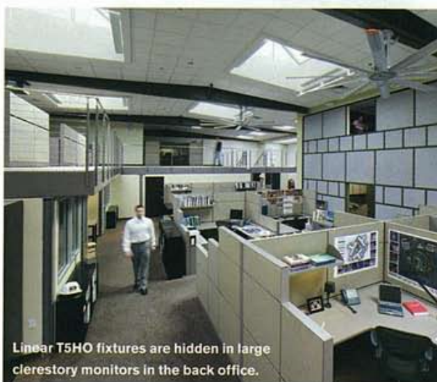
Workstations in the front of the building are lit by custom hybrid daylight and fluorescent troffers.
